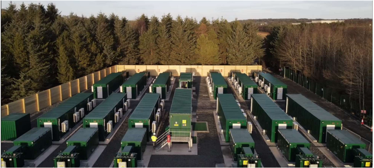
Figure 1 Example of BESS Site at Byers Brae, Scotland
